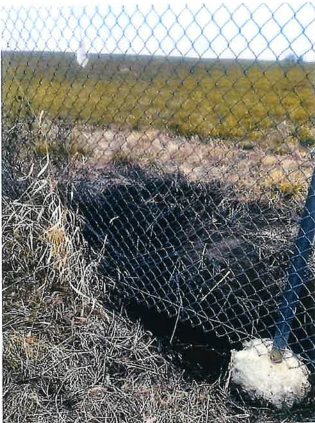
East fence tile blowout getting worse.
