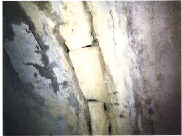
Blocks that once backed mortar joint
