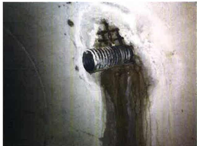
Rebar impacted with underdrain
