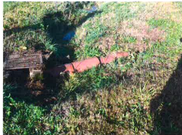
Failing structure, tile and ditch
