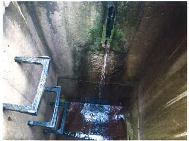
Overactive underdrain due to lack of crack sealing
