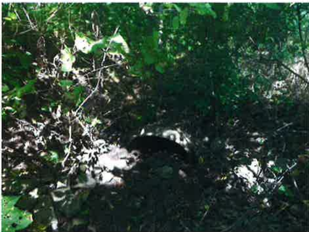
Obstructed outlet in the 100-year floodway south of the airport
