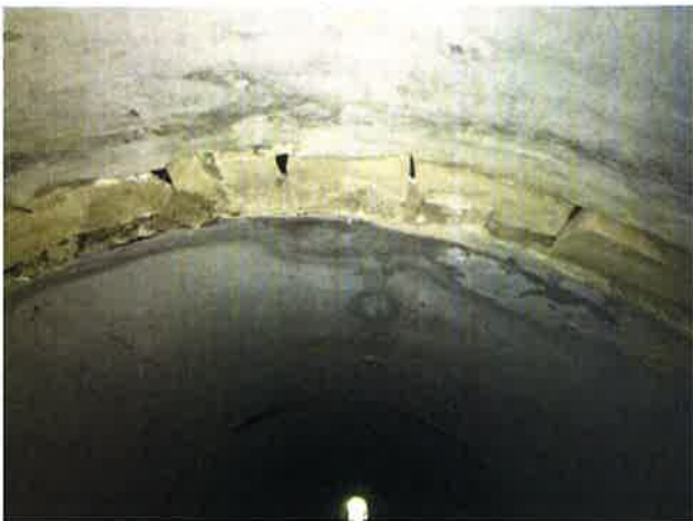
Blocks that once backed mortar joint
