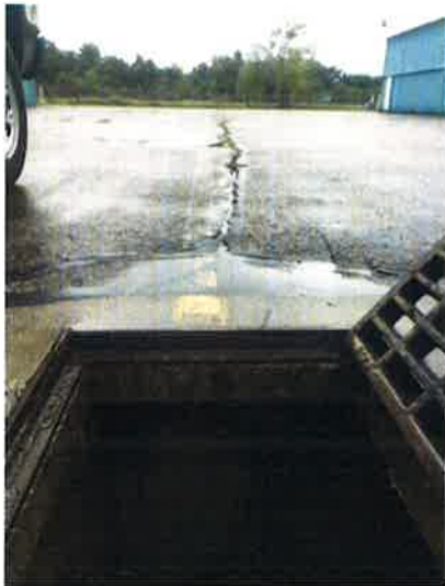
Crack serving as a trench drain
