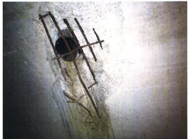
Rebar impacted with underdrain
