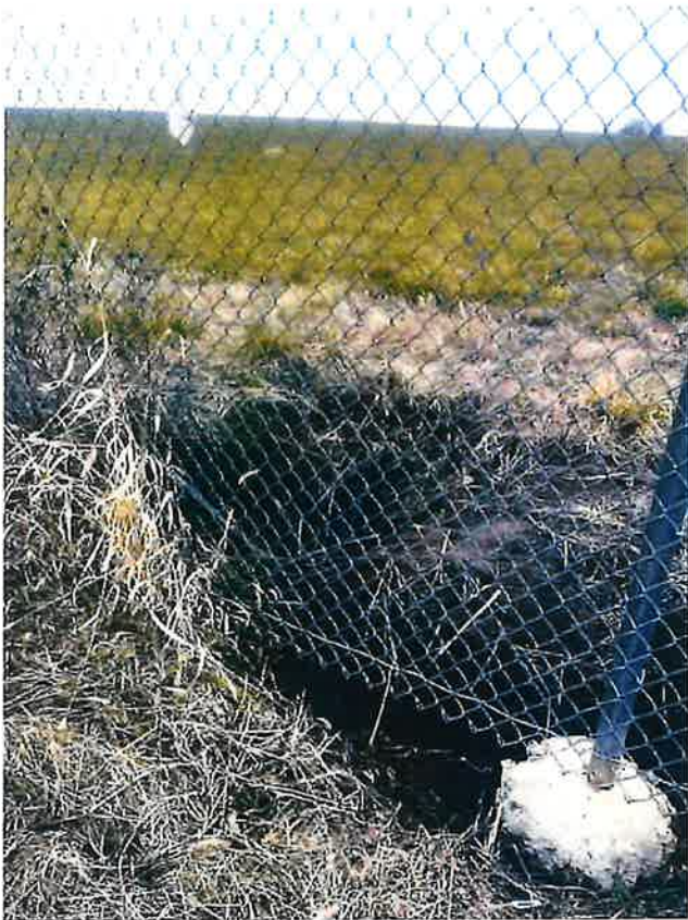
East fence tile blowout getting worse.
