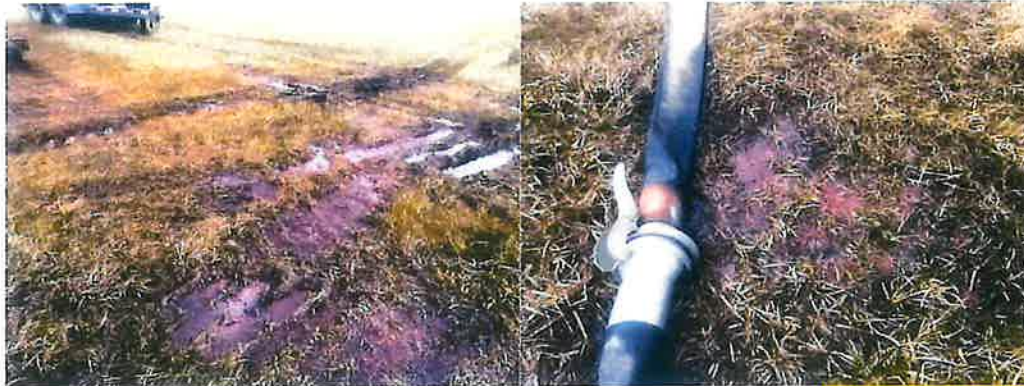
Diesel on the ground near taxiway/runway culvert replacement. Clean-up ASAP.
