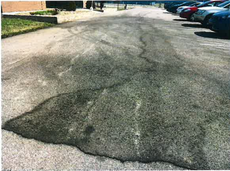
A-Assumed Parking Lot Spill
