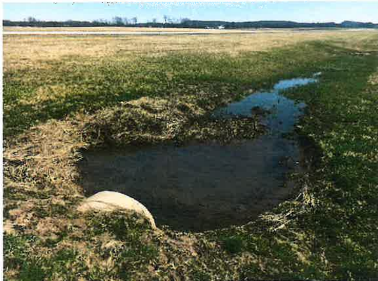
B-North tile overflow to taxiway culvert overflow. Flow is strong several days past recent rain.
