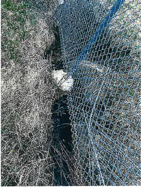
Sink hole on outer edge of airport fencing.
