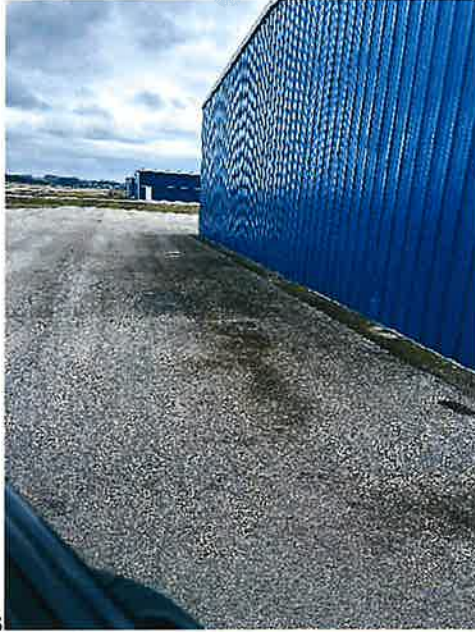
Staining outside of hangars
