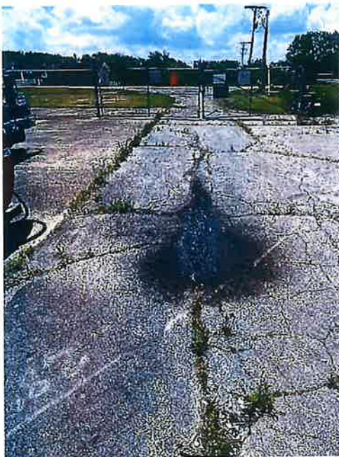
Spills appear to be increasing at the remote fuel island.
