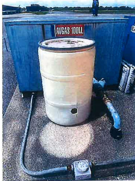
Hole in spill barrier container.
