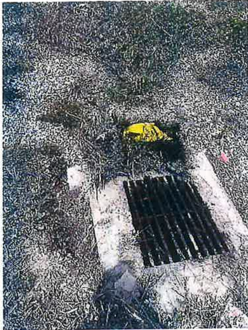
System #2 infield drain covered
