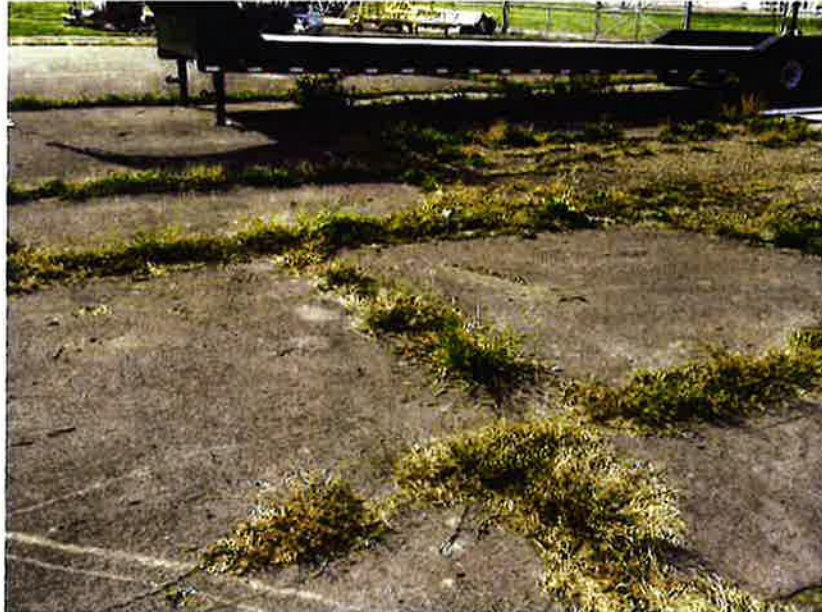
Figure 11. Weeds and grass growing within cement pad and apron.
