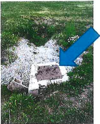
System #2-needs regular cleaning
