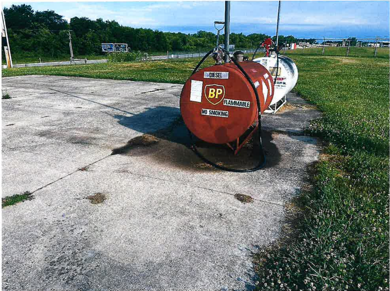
Fuel spill stains at 3383 Old Columbus Road.
