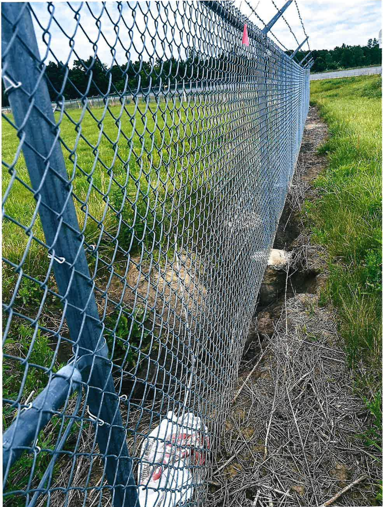
Repair failed tile and erosion at Election House Road fence indentation.
