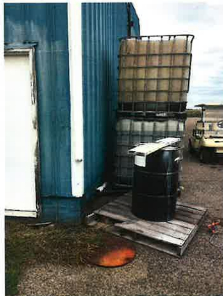
SE Corner Building J-Downspout missing
